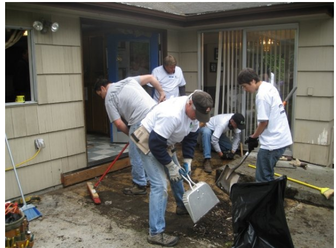
Volunteers from the Adobe, Panattoni, IFMA, and Kibble & Prentice teams demolish and build a new deck for the residents of a Parkview Services home in Lake City.
